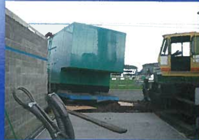
Placing the generator on the new pad required removal of fencing and maneuvering the unit as close as possible to the pad in order to avoid power lines during the lift.
