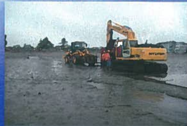
On May 26, 2010 The repairs began on the outfall that was installed in 1956,
