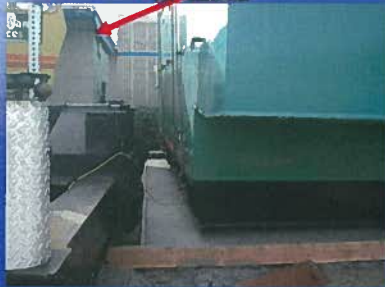
Tolerances were tight and had to be exact to allow room for enclosure doors to open. Notice the building's eave, which had to be modified.
