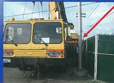
The large crane required to do the lift had to be placed perfectly to allow rotational movement. The fence had to be pushed out a few inches. You will notice a 2x8 supporting the fence and distributing the pressure.
